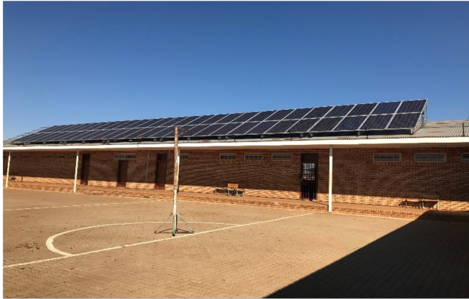
Solar PV System
