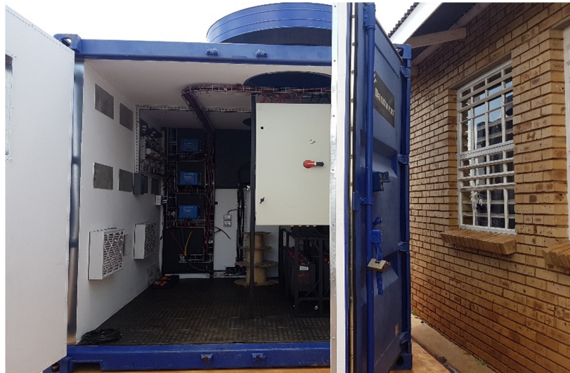
Power Management System and Battery Storage
