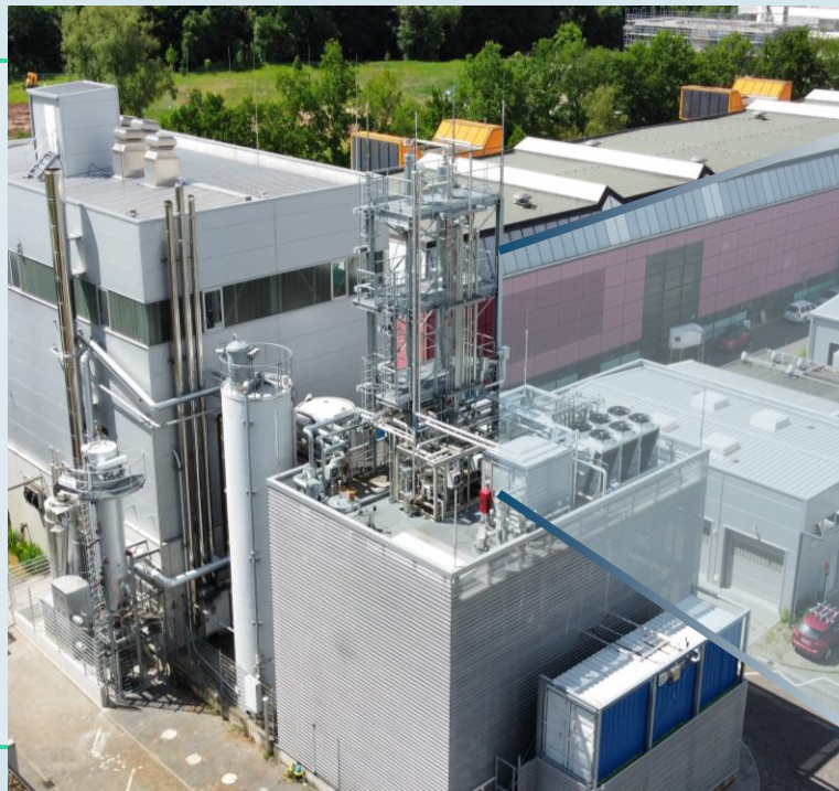
HTW® facility at TU Darmstadt (Energy Systems and Technology)
