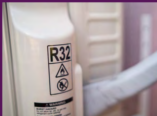
R32 is a lower global warming potential (GWP) F-gas refrigerant
